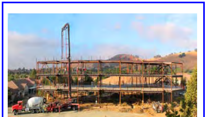
The new assisted living building progresses. Soon Estates Drive will be paved and available for traffic.
