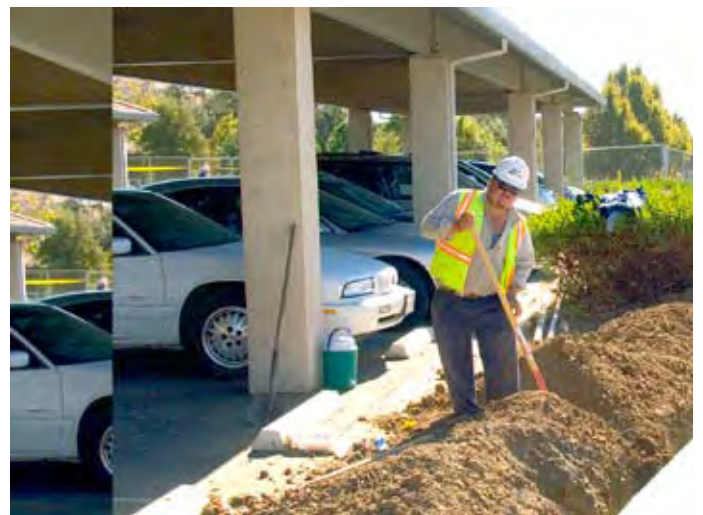
Irrigation pipes for new landscape planting are being installed in front of Building 2000.
